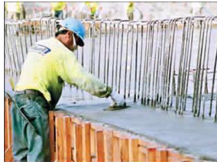
Twenty three million pounds of concrete were distributed over 15 hours—the largest concrete placement in the Coachella Valley to date.
